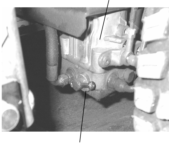
Bypass Valve (one on each hydrostatic transmission)
